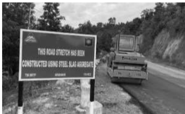
Road Stretch of Joram-Koloriang Road constructed using Steel Slag, Source: BRO images
