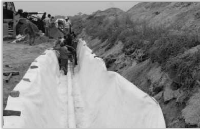
Sub-Surface Drainage System at Barrackpore Runway, Source: BRO images
