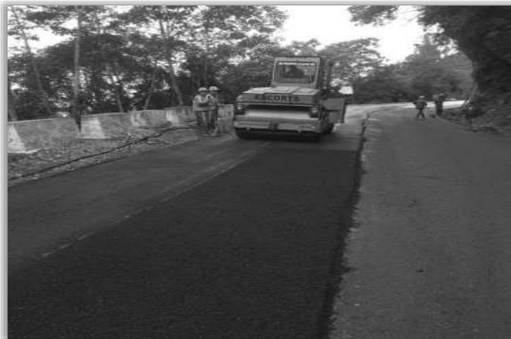
Resurfacing using plastic waste on Phuentsholing–Thimphu Road in Bhutan, Source: BRO images
