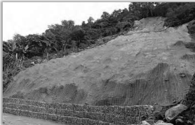
Biodegradable Coir reinforced with Gabion Wall on TCC-Maza Road, Source: BRO images
