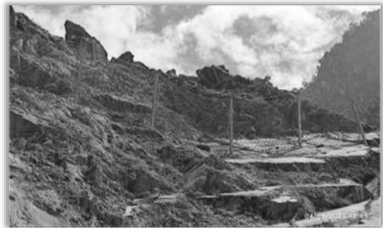
Dynamic Rockfall Barrier on Joshimath-Mana Road in Uttarakhand, Source: BRO images
