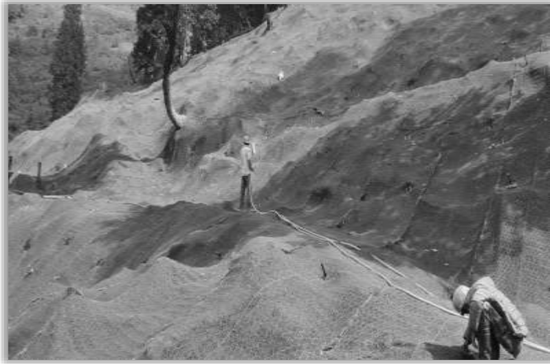
Reinforced Geomat on approach to South Portal of Atal Tunnel, Source: BRO images
