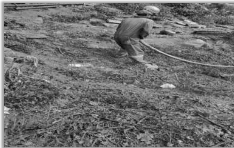
Hydro Seeding on approach to South Portal of Atal Tunnel, Source: BRO images
