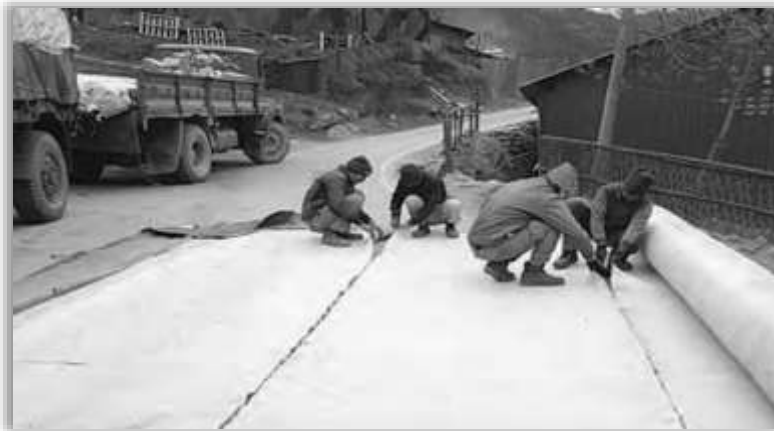
GCCM being prepared to make drains along road TCC- Taksing, Source: BRO images
