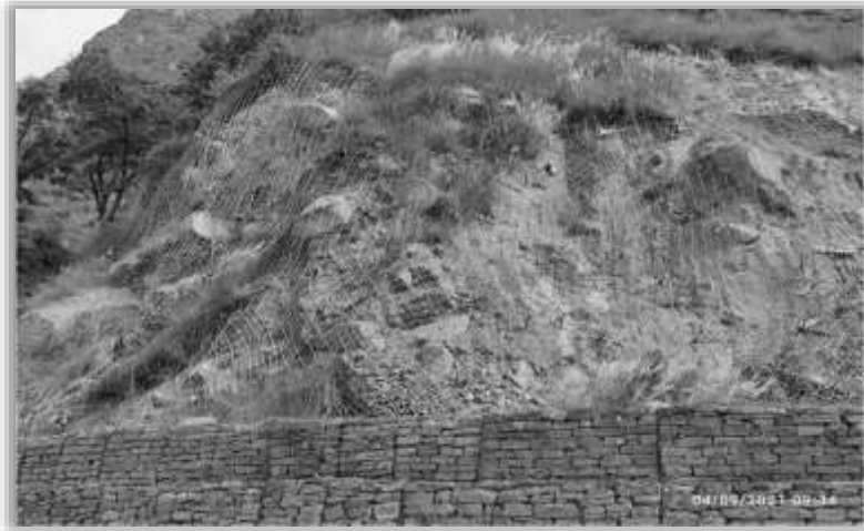
Drapery with Hill Side Gabion Wall on Joshimath-Mana Road in Uttarakhand, Source: BRO images
