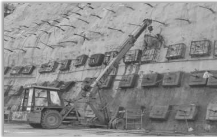
Pre-Stressed Cable Anchor on approach to South Portal of Atal Tunnel, Source: BRO images
