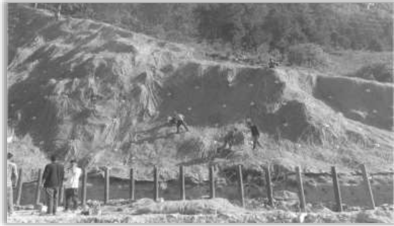
Secured Drapery with Micro Piling Work on Joshimath-Mana Road, Source: BRO images
